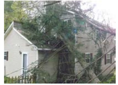
Snowstorm damage at Camp O'Cumberlands
